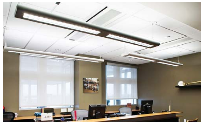
Greenspun Hall, UNLV, Las Vegas, Nevada DID302 active chilled beams
